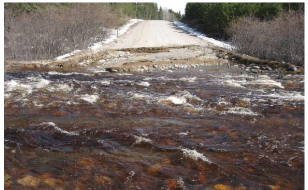
Figure 1. Designing resource roads and infrastructure to resist all climate events is not practical or economically feasible.
