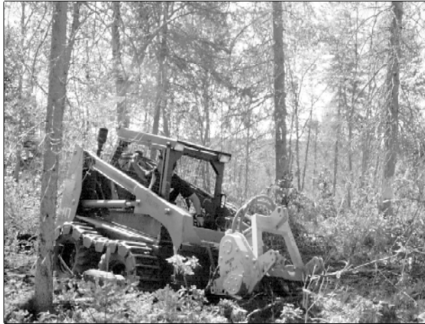
Figure 3. Mulching with the Meri Crusher MJ-0.8 mounted on a Thomas HD233 skid-steer loader.
